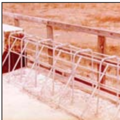
At a construction site, galvanized, fabricated rebar has been installed and is ready for concrete to be placed.
