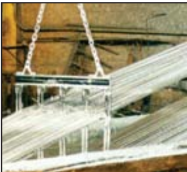
Rebar being removed from the molten zinc bath. Excess zinc runs off the bars, but enough zinc has bonded to the steel to protect it from corrosion for decades.
