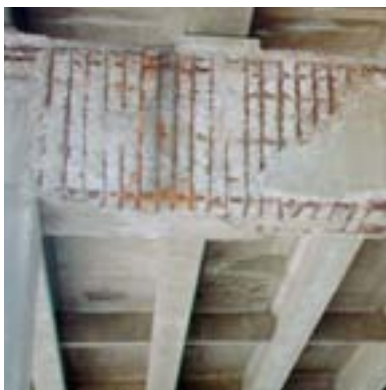
Corrosion of unprotected reinforcing steel creates hazards due to spalling concrete.
