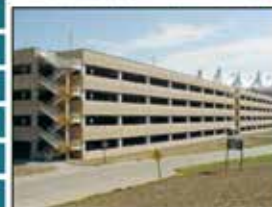
Painted Parking Garage Stairs after 8 years of service
